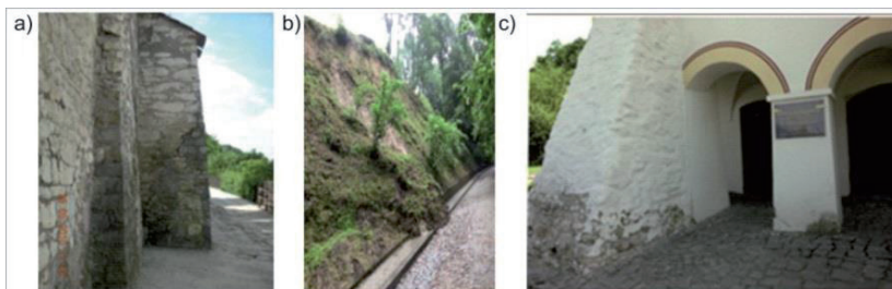
Fig. 14: a) Poorly renovated medieval opokas walls; b) retaining wall unprotected from rain, moisture and slides; c) poorly medieval renovated granary
