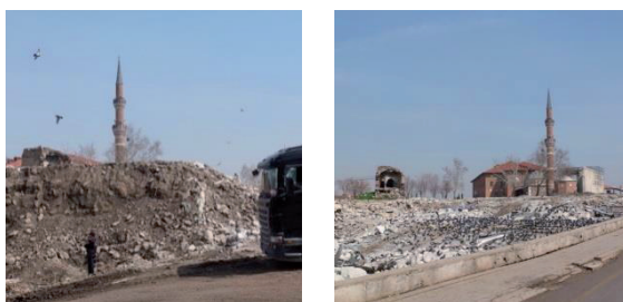
Figure 7: Hacı Bayram District Under Construction for the implementation of renewal project. Source: A. Güliz Bilgin Altınöz
