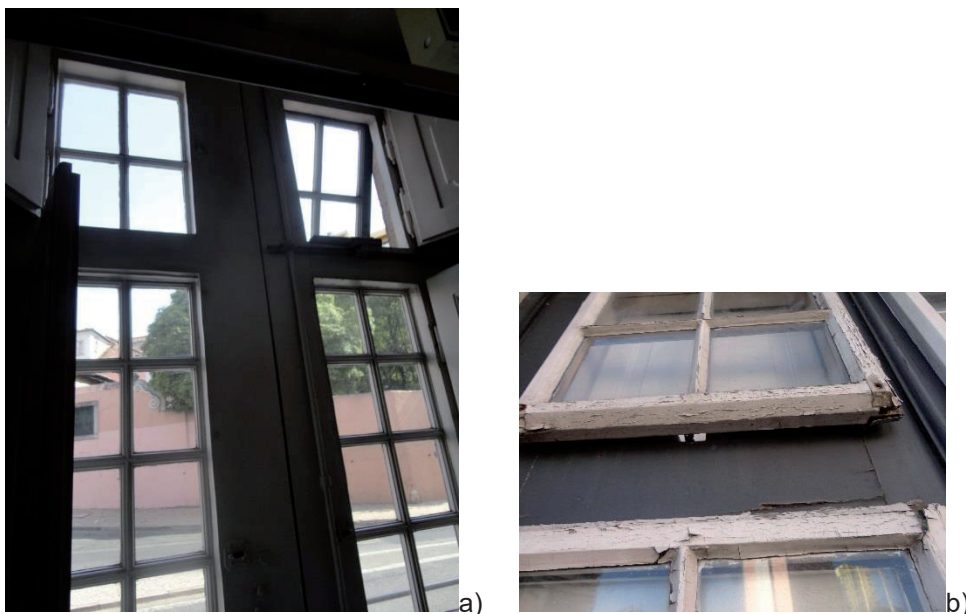
Figure 5: Windows for natural ventilation. a) projecting leaf at top, b) small projecting opening in the leaf
