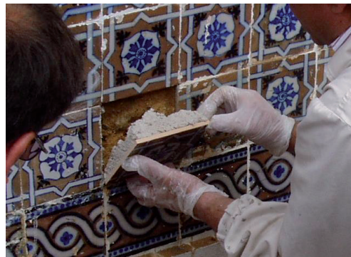
Figure 8: Repair of Azulejos façade cladding with air lime reattachment mortar by a skilled applicator (conservator / restorer)
