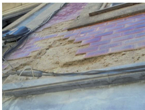
Figure 2: Azulejos cladding in a housing building façade with degradation due to loss of cohesion of bonding mortar (Porto, Portugal)
