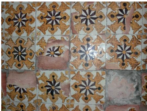
Figure 7: Azulejos façade cladding repaired with cementitious reattachment mortar showing degradation due to salts and high stresses
