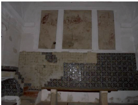
Figure 3: Azulejos cladding of interior wall panel with degradation (loss of cohesion) of bonding mortars due to moisture (Church).
