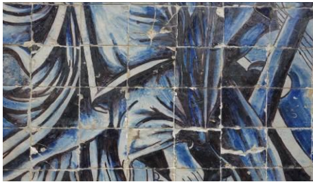
e. Surface cracking / glazing release.
