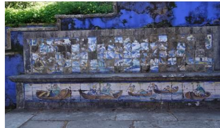
d. North side exposure deterioration.
