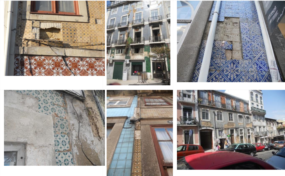
Figure 2 – Degraded tile facades
