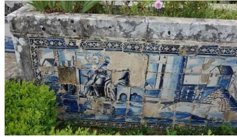
b. Humidity/ water infiltration.
