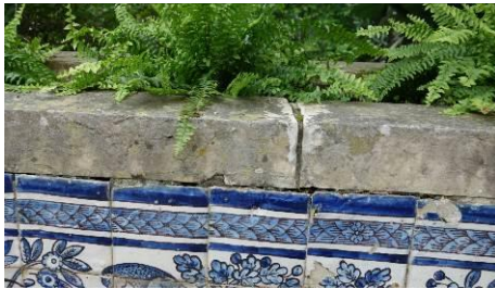
c. Open masonry joints.
