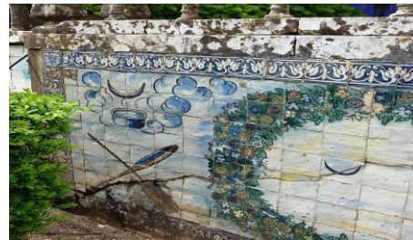
b. Panel fracture – masonry wall rotation.
